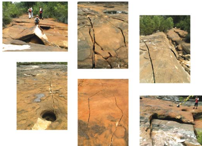
Julie Sheppard, 'Waratah Rivulet: Cracked, Drained, Polluted', 2007. The Waratah Rivulet makes up about 30% of the Woronora Dam catchment. The Rivulet is dry because of the impacts of underground longwall coal mining 500m below the surface.
